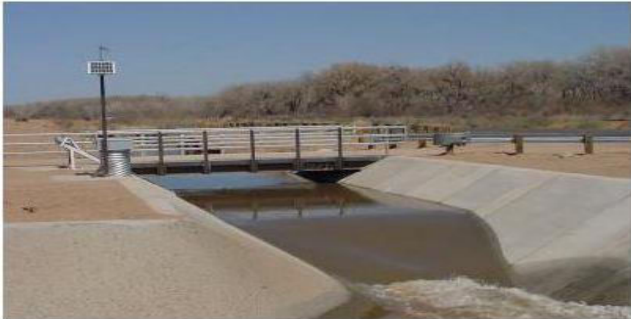
Broad Crested Weir & Gauging Station
