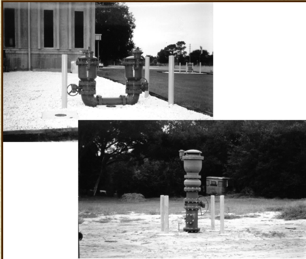
Water supply wells, Floridan Aquifer near Tampa, Florida
