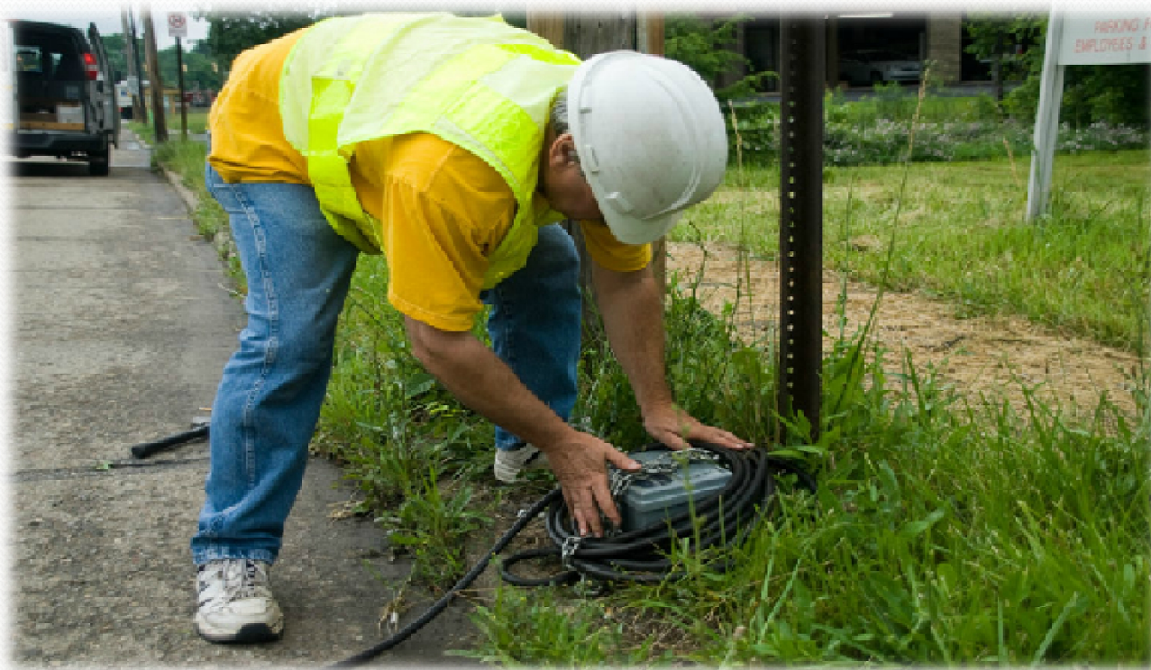
Figure : Pneumatic Road Tube
